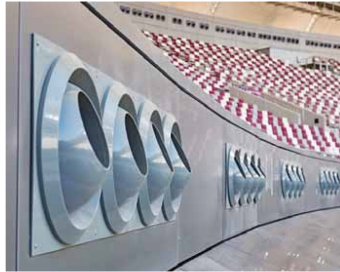
Plastic nozzles are an integral part of Qatar's stadium cooling technology.
